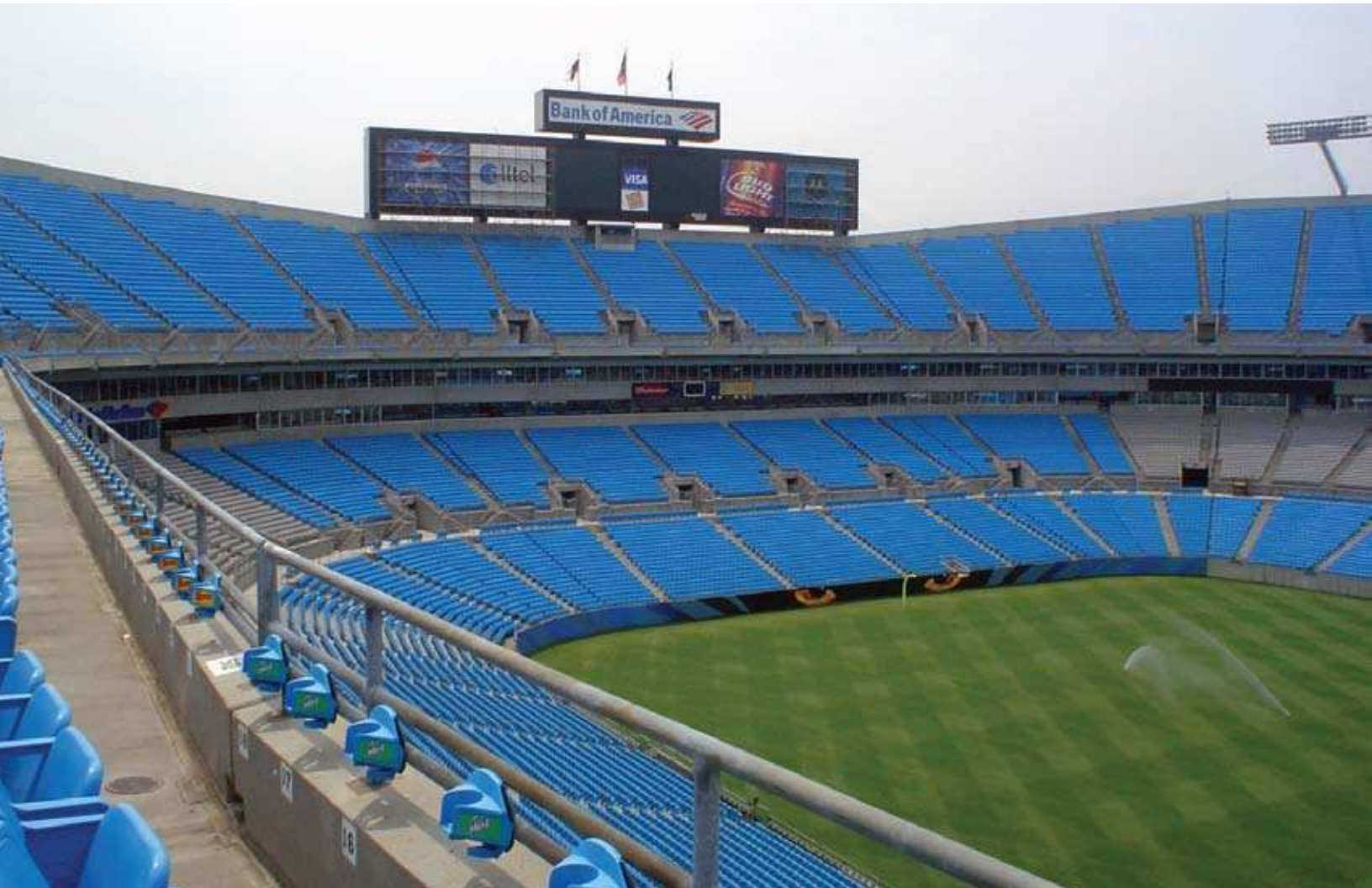
ProSpec Vinyl Concrete Patcher and 118 Primer were used for concrete repairs at Bank of America Stadium in Charlotte, North Carolina.
