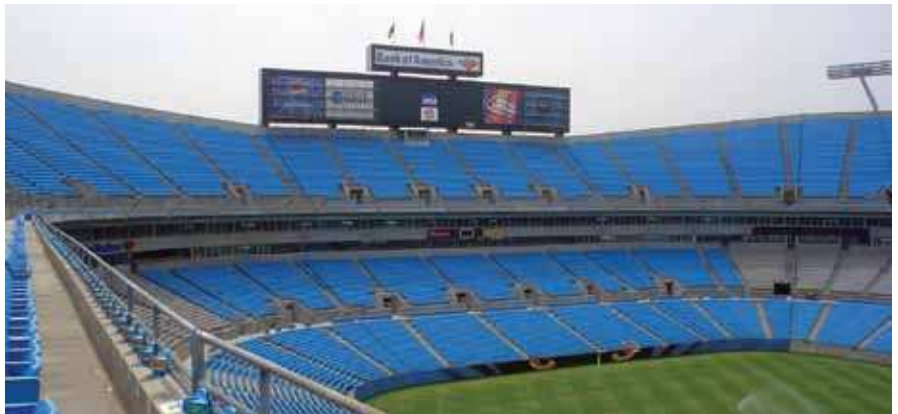
ProSpec Vinyl Concrete Patch and 118 Primer were used for concrete repairs at Bank of America Stadium in Charlotte, North Carolina.
