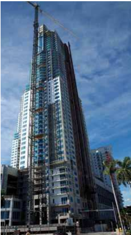
Everglades on the Bay in Miami, Florida, a luxury condominium project, used ProSpec Vertical Leveling Mortar to repair out-of-plumb walls, preparing them for a stucco finish coat.
