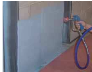
Barritech VP spray-applied in a single coat at 60 mils wet on concrete block
