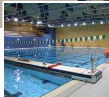
Fry Reglet Baffle Panels installed in the rafters help control sound in a large indoor pool area.
