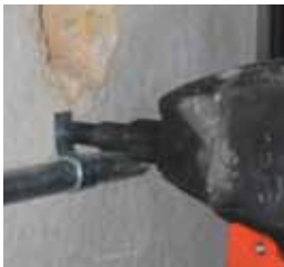
12HSMP034 clip assembly used to secure conduit
