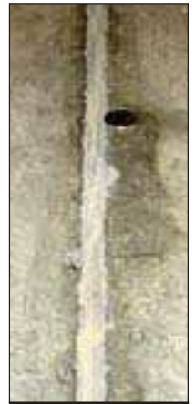
Ex. Finished Area
