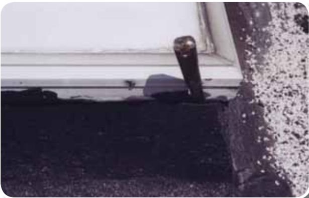
Skylight with membrane pulled away from counterflashing.
