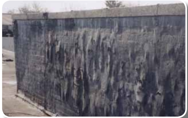
Cracked concrete coping cap, allowing water to infiltrate the painted brick wall.
