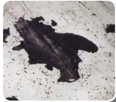
Worn coated roof surface.
