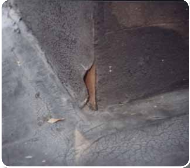
Open lap at Roof Top Unit curb.
