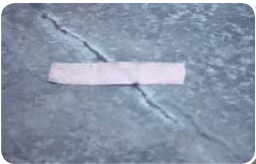
Improper roof repair.
