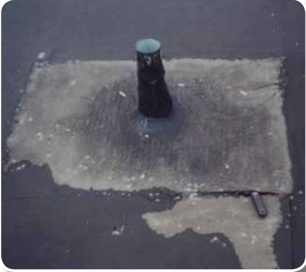
Open lap at target patch at Vent Thru Roof.
