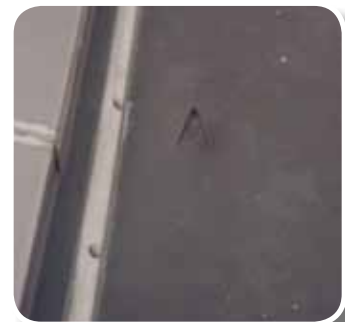
Gouges in a roof membrane.
