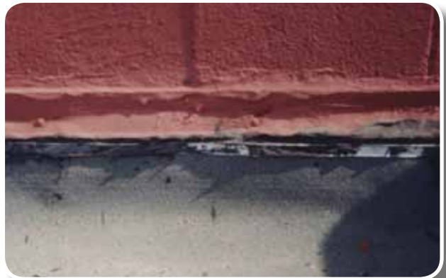
Membrane and counterflashing pulled away from brick wall.
