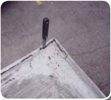
Coated roof pulled away from edge.
