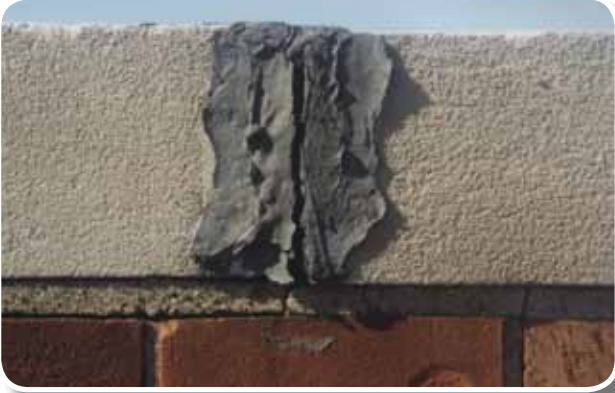
Brick Coping Cap with aged and cracked sealant.
