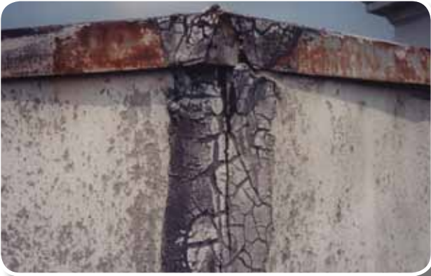
Rusty Edge Metal deteriorating, allowing moisture to migrate into roof system.
