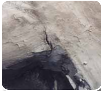
Cracked coated roof.
