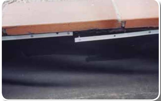
Termination Bar with fastener pull out.
