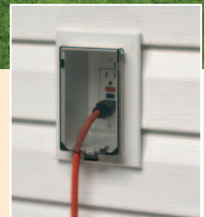
Recessed Electrical Boxes
