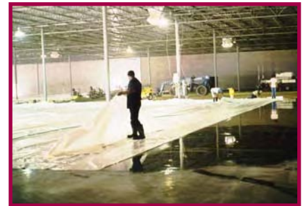
Place Transguard® covers so they lay flat, with a minimum 6" of overlap.
