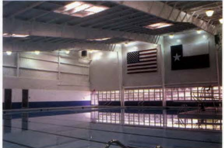
The effects of high humidity and exaggerated differences in interior/exterior vapor pressures associated with indoor pools can be controlled with an effective vapor barrier system.
