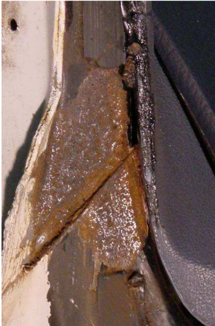
(Level 2 – 3 corrosion of pinchweld)
