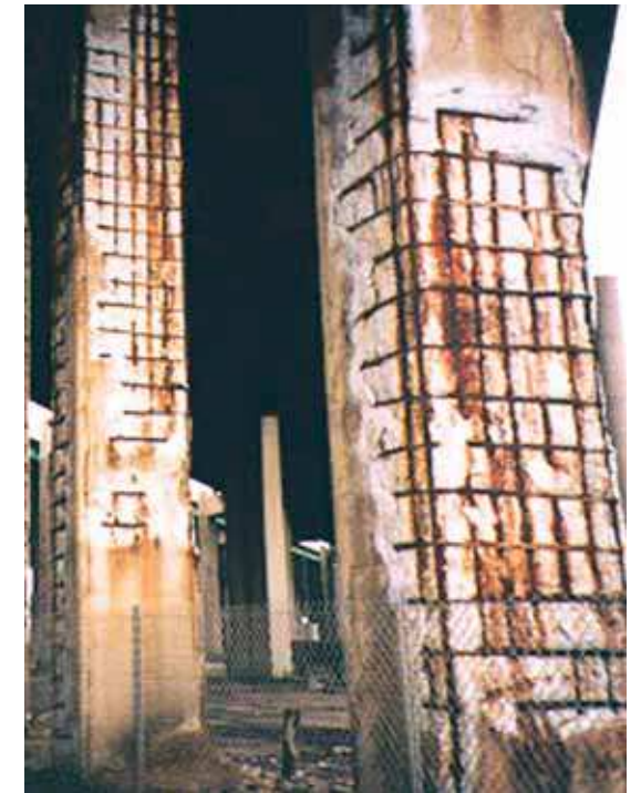
These bridge columns had to be demolished and rebuilt because the corrosion was too far advanced.
