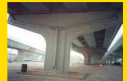
Case study provided by Vector Corrosion Technologies.
