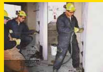
Case study provided by Vector Corrosion Technologies.
