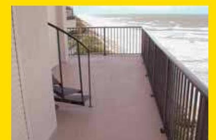
Case study provided by Vector Corrosion Technologies.
