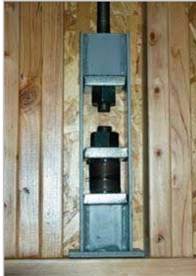
Previous Anchor Tiedown System
