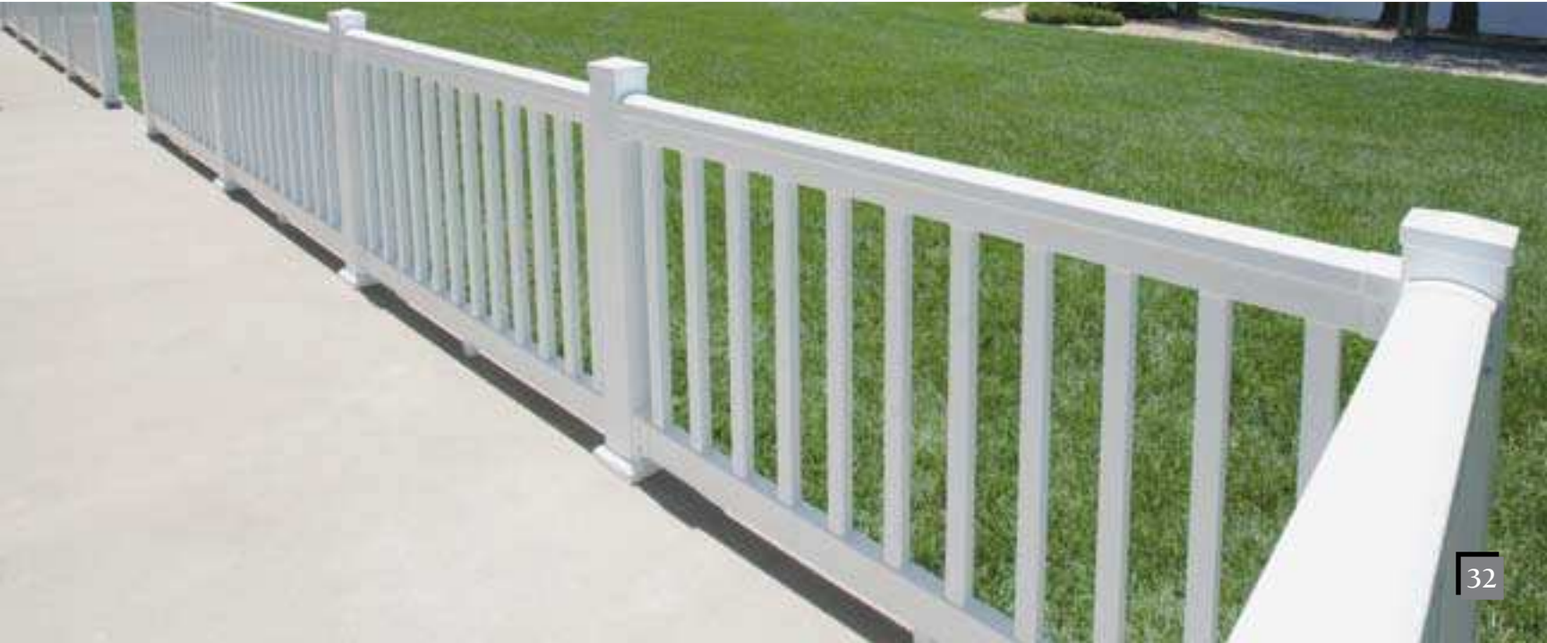
Railing color is White. Photo of actual deck in Carl Junction, Missouri.
