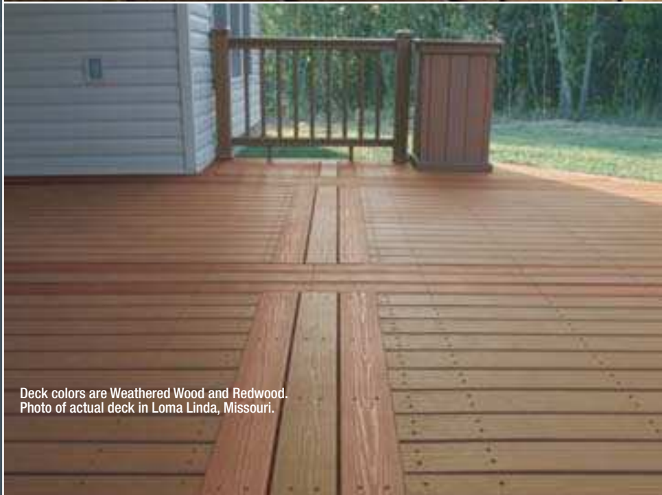
Deck color is Weathered Wood. Photo of actual deck in Joplin, Missouri.
