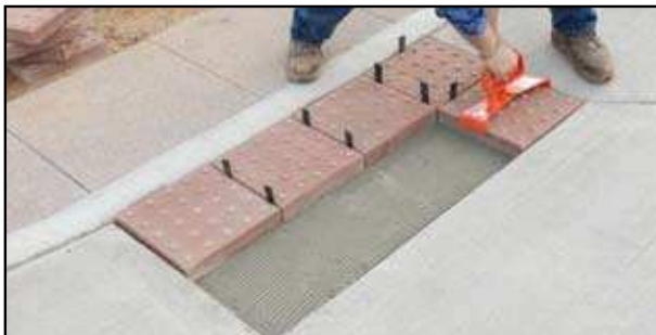
Step #3 - Thin Set Installation - Set pavers. Be sure pavers are fully set into thinset. (Back buttering may be necessary.)
