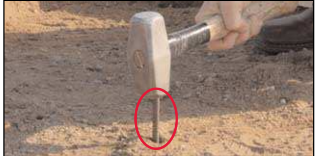
2- Drive in rebar to the approximate height to receive Wausau Tile's block-out frame. The framework has small feet to help locate where rebar should be located.
