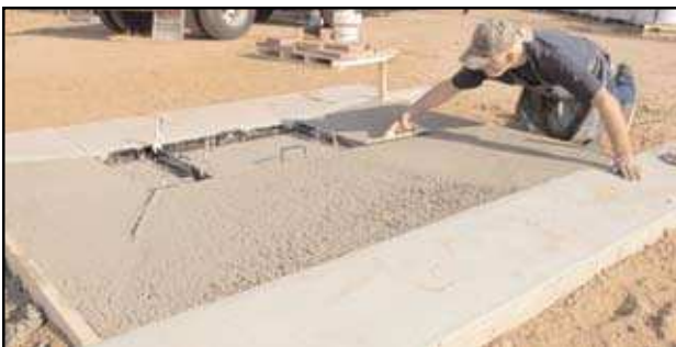
5- Pour concrete into and around framework. Level concrete and bull float area.
