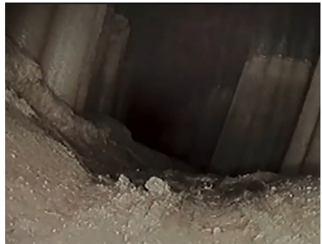
Sediment in tank
