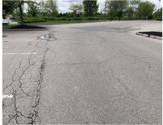
Example of pavement distress
