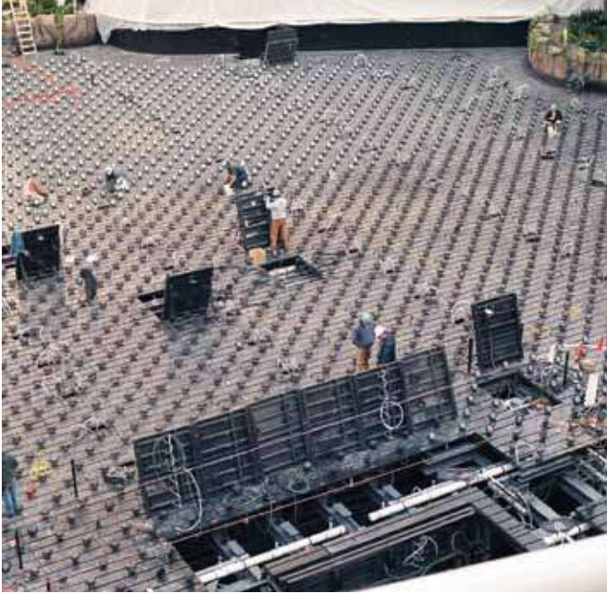
Custom FRP Water Features
