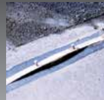
Leaking Flashings & Penetration
