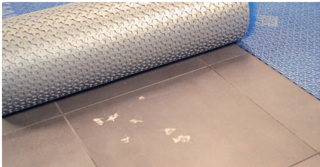
Existing cracked tile
