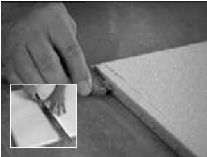
Tegular-edge border panels may require field cutting. Cut border panels face up and paint edges
