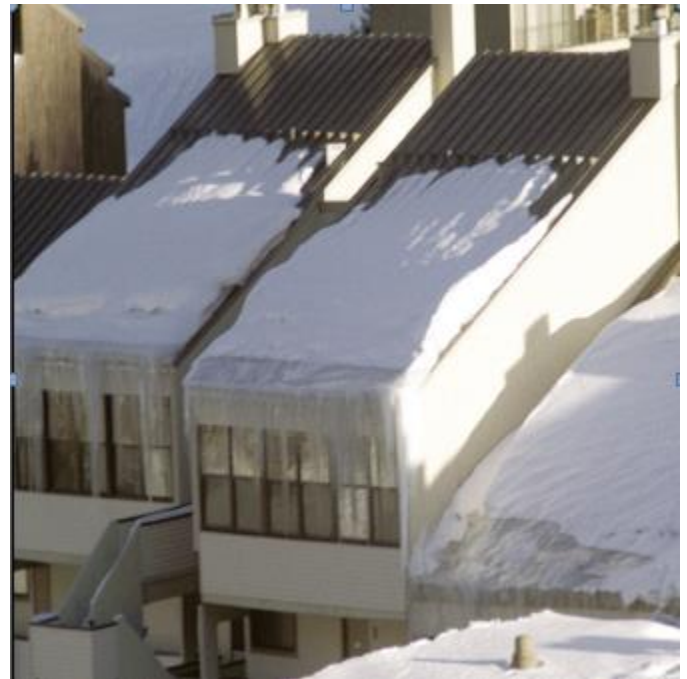
Figure 6B: Ice dams create unintentional snow retention
