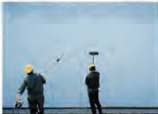
Figure 1. Effect of cleaning dirt off a building
