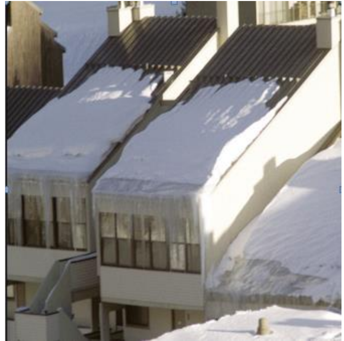
Figure 6B: Ice dams create unintentional snow retention
