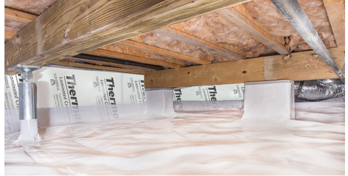
Crawlspace with ThermalStar LCI
