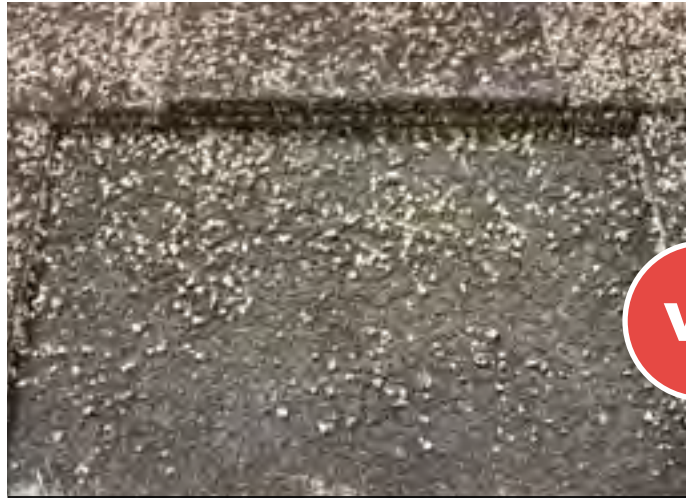
Standard Asphalt Roof With Severe Granule Loss
