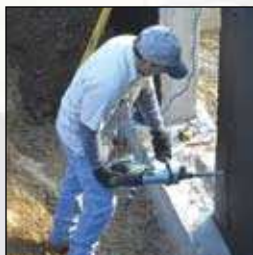
1. The foundation opening is prepared to receive the PermEntry casting. Holes for the special high-strength bolts are drilled through foundation.
