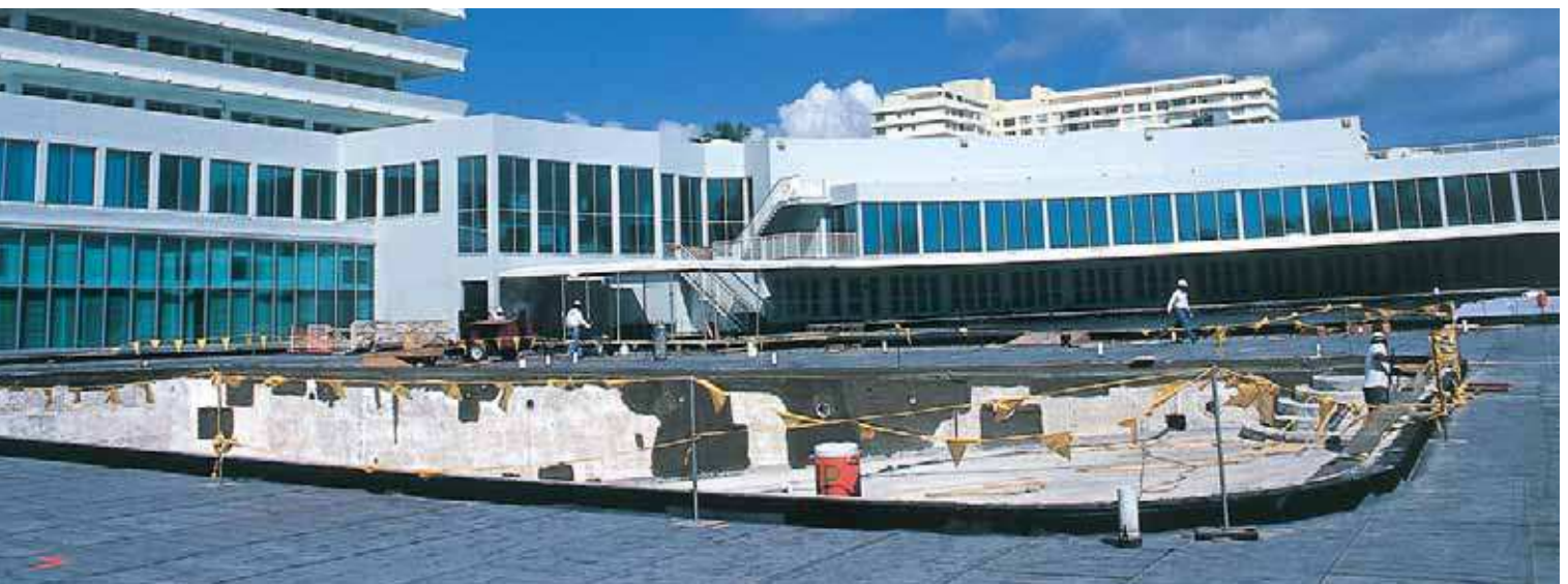
With the pool deck nearly ready for bricklayers, Pro-Tech crewmembers work to ready the area for a leak test — in this case, complete immersion in four inches of water for 48 hours. The rubberized asphalt decking system passed with flying colors.
