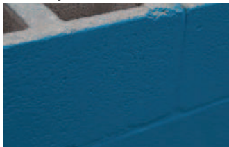
Coating A, Below Specified Thickness
