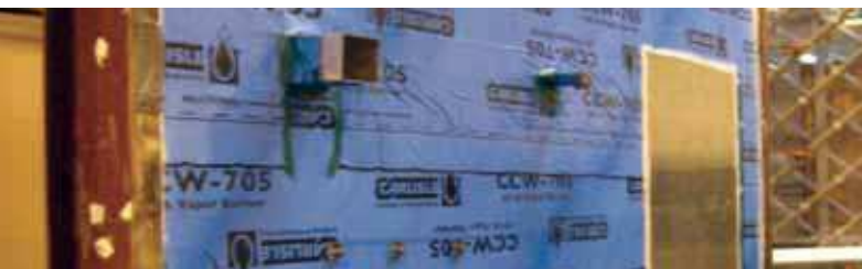
CCW-705 Self-Adhering Membrane Mockup (Specimen #2)
