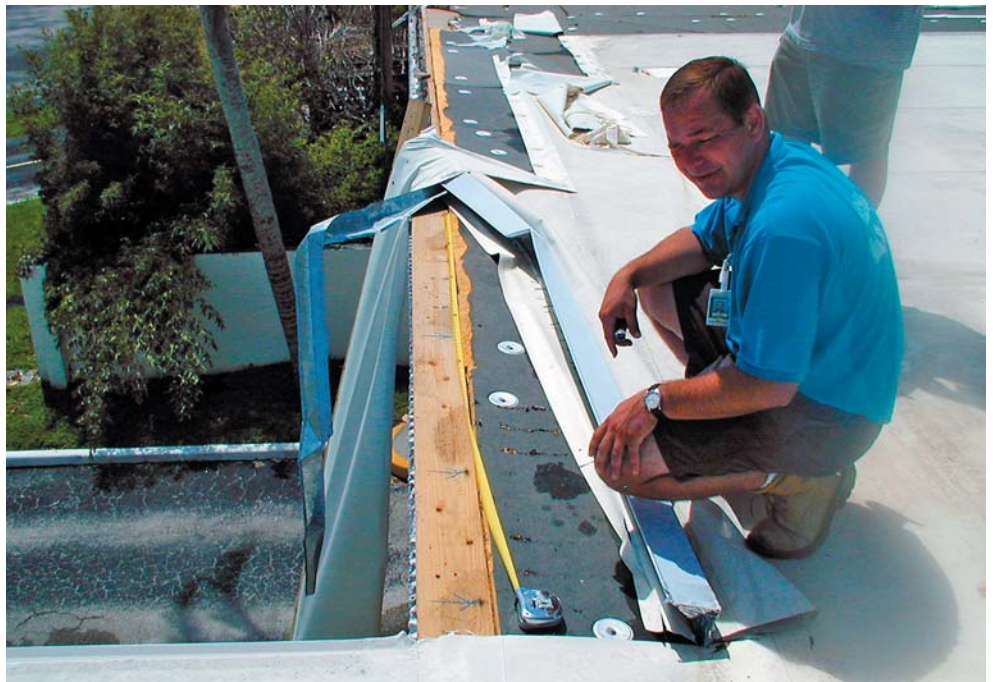
Charlotte County South Annex: Enhanced attachment of nailers and metal work would have likely allowed this roof to fare much better. Photo courtesy of RICOWI
