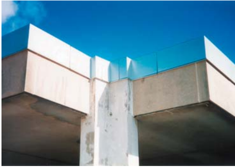
Many paints will not hold up to the extreme UV exposure roof edges endure. An old roof edge (top) at Conrad Hall at Michigan State University was replaced with a new system (bottom).
