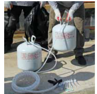
Shaking of A-side and B-side tanks
