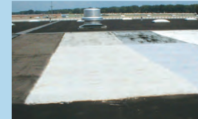
FlintCoat-W and FlintCoat-A after five years in service, with and without FlintCoat-E.
