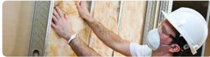
CertaPro™ Commercial Insulation
