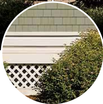
Multiple profiles used in water-table application and skirting.
