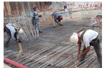
POST INSTALLATION DAMAGE
