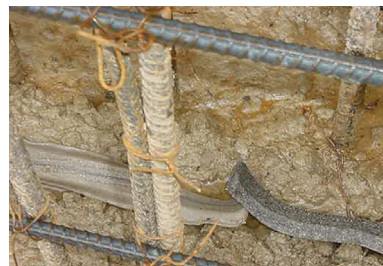
BAD INSTALLATION AND DETAILING
