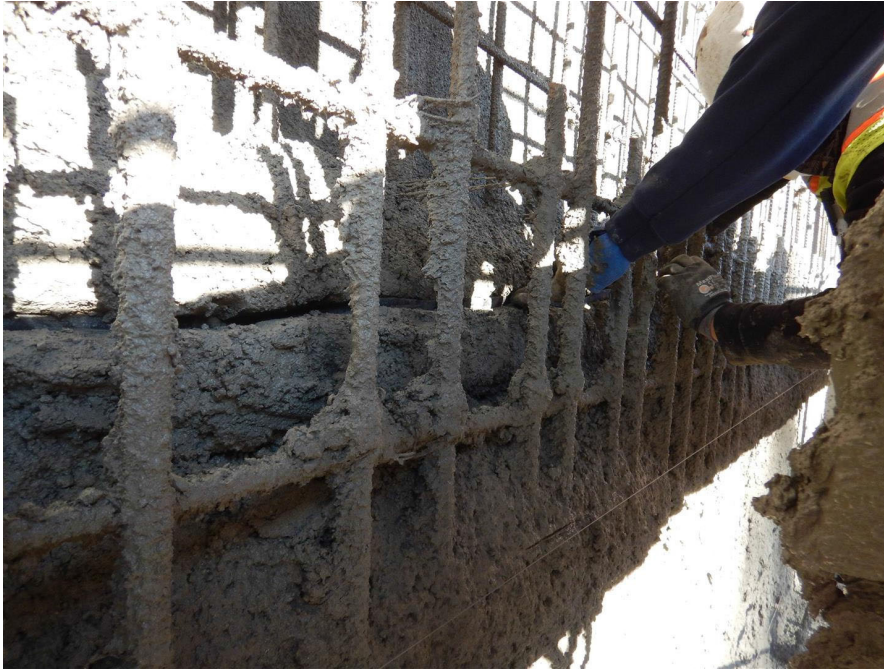
PHOTO 1: SHOTCRETE LIFT JOINT
