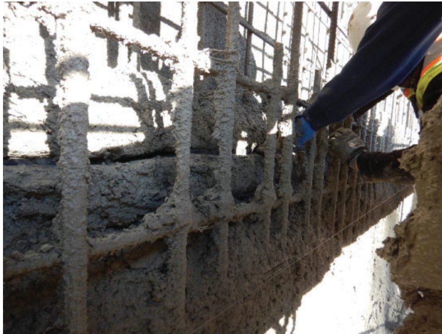
PHOTO 1: SHOTCRETE LIFT JOINT
