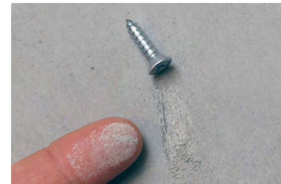
Non-densified concrete easily erodes and dusts.
