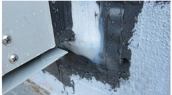
Figure 4: Sealant attaching strip and corner to air barrier in-field. Lap joints sealed.
