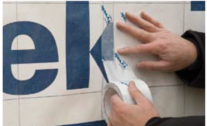
Taping the seams after wrapping is the best practice for completely sealing the building envelope.
