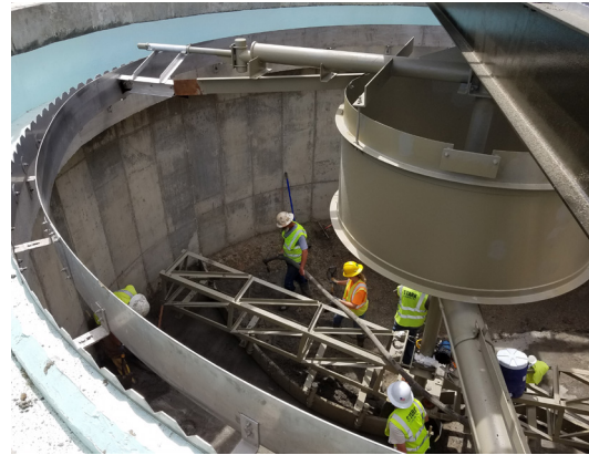
RESURFACER BEING PUMPED AND INSTALLED. NOTE THE USE OF THE SLUDGE RAKE AS A FINISHING TOOL.
