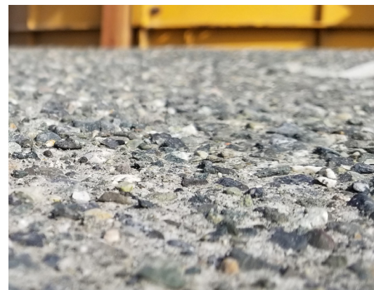
SURFACE PREPARATION USING A "SURFACE RETARDER". ADDITIONAL SURFACE PREP MAY BE REQUIRED TO ACHIEVE CSP10.
