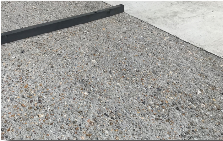
PROPERLY PREPARED FOUNDATION SURFACE FOR EPOXY GROUTING. FOR EXPANSION JOINTS, REFER TO SECTION E.
