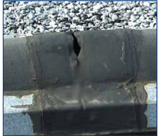
Splice Failure on Competitor's product
