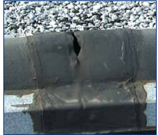
Splice Failure on Competitor's product
