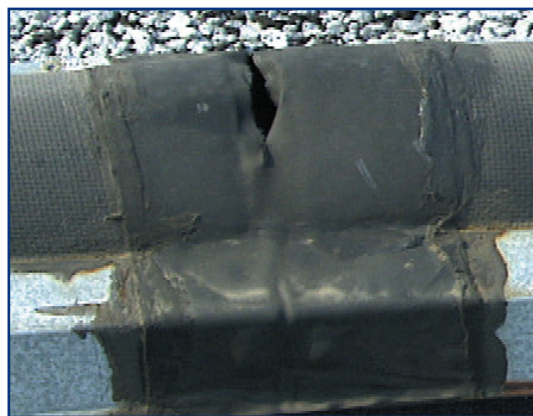
Splice failure on competitor's product
