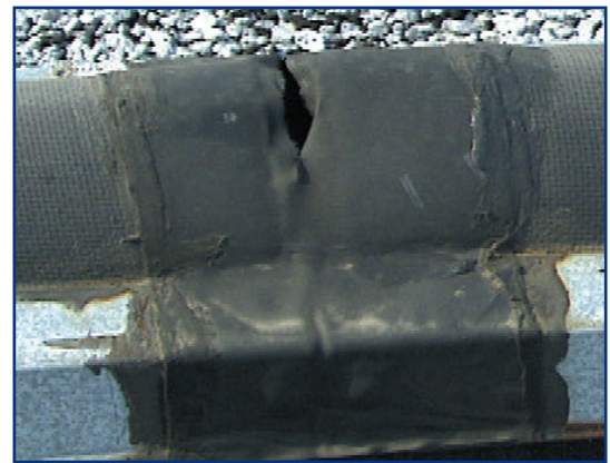
Splice failure on competitor's product
