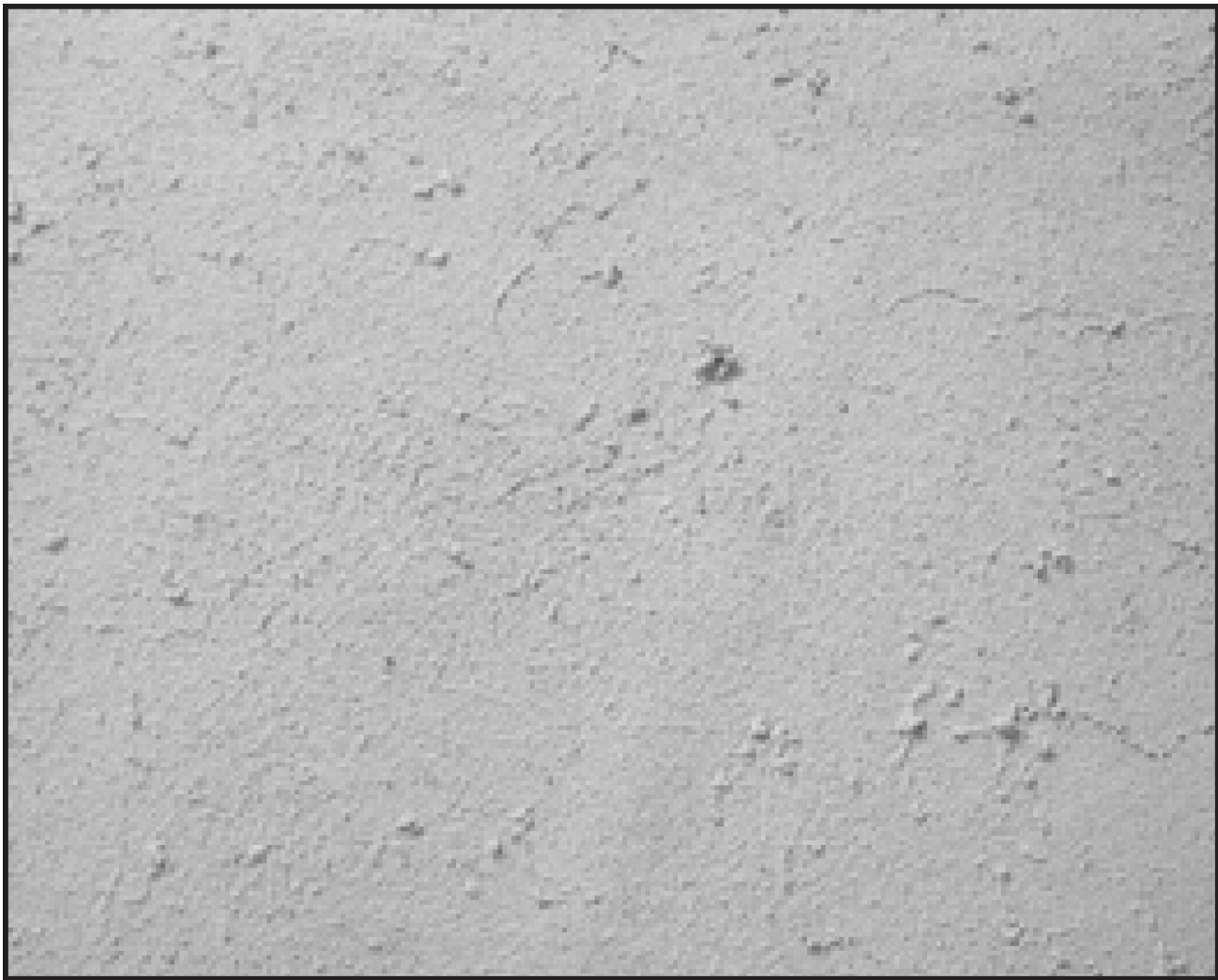
Photo 2. Example of over-mixing.
