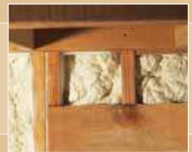
SELF-ADHESIVE SPRAY SEALS SMALL, TIGHT SPACES, UNDERSIDE OF ROOF SHEATHING AND FLOOR BOARDS.
