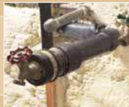
SEALS PIPES AND THROUGH-THE-WALL PLUMBING PENETRATIONS.
