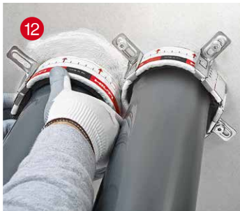
12 Piping and ventilation
