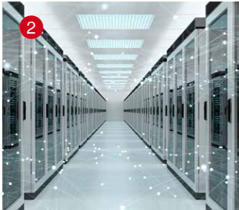
2 Hot / Cold aisle containment
