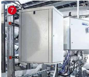
7 Equipment supports and platforms
