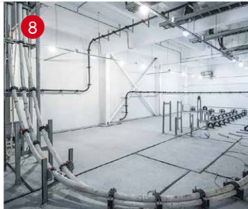
8 High-voltage cabling supports
